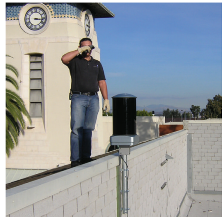
ClearMesh 300s are rooftop mounted and connected to up to 3 different buildings within the mall campus to create a highly resilient mesh network.
